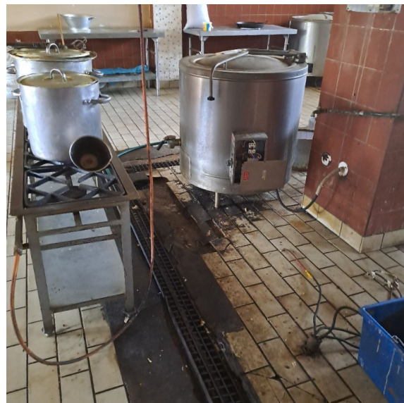
Figure 9: Kitchen Appliances (faulty), Police Station Windhoek Central
