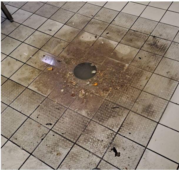
Figure 8: Kitchen Plumbing (blocked), Police Station Windhoek Central
