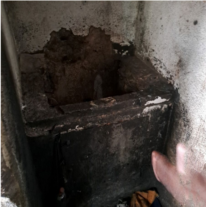
Figure 6: Handwash Basin, Police Station, Windhoek Central
