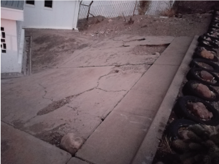
Figure 16: A retaining wall destroyed by drainage, causing further destruction to the drainage channels below
