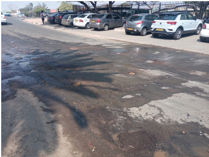
Figure 15: Improper drainage destroying a local road
