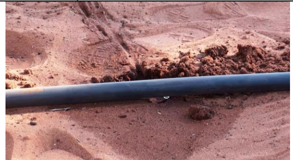
Water drips from one of the outlet holes.
