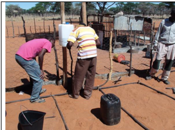
A drip irrigation system is installed in the garden.
