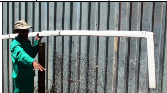
A gutter and down-pipe will lead rainwater from the roof into the compost pit garden.
