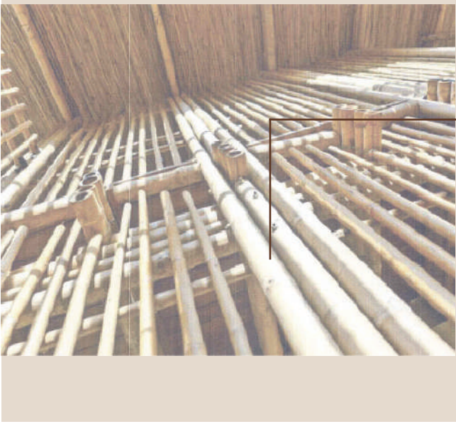
Figure 109: Bamboo beams (Rakz, 2014)
